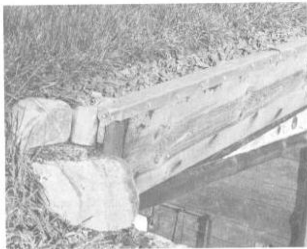
Illus. 15-2. Removing the sod within 5" of the retaining board and replacing it with a layer of sand covered by 6" of crushed stone improved the drainage and relieved the lateral pressure from the retaining board.
