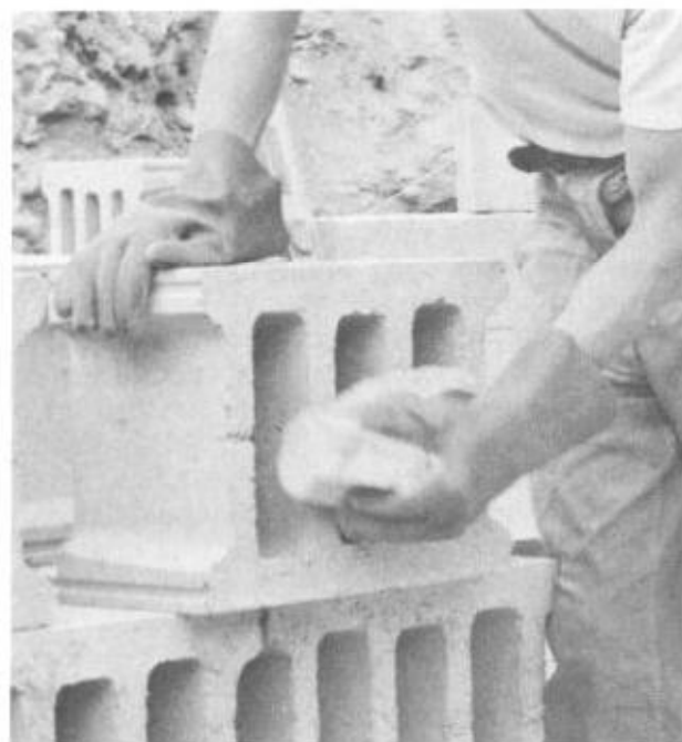
Illus. 6-1. Before stacking, a piece of broken block can be slid across other blocks to knock off excess materials and burrs.
