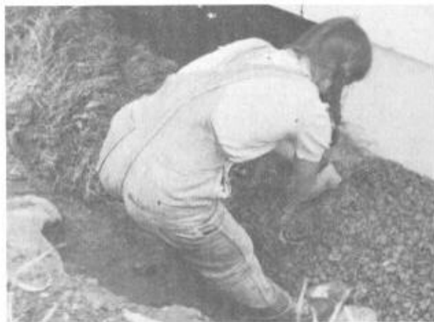
Illus. 10-5. Hay spread on top of the stones covering the footing drains will decompose and form a mat to stop infiltration into the drain by the subsequent sand backfill.
