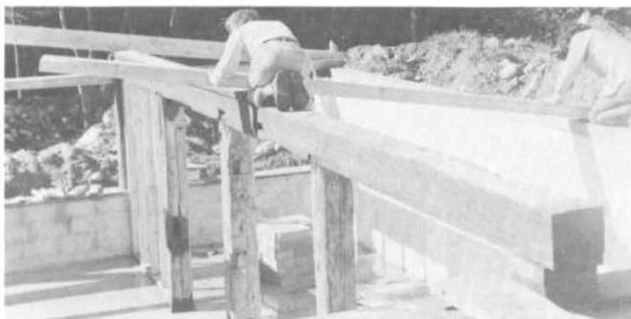
Illus. 7-7. The rafter is slid along the beams and put into position.
