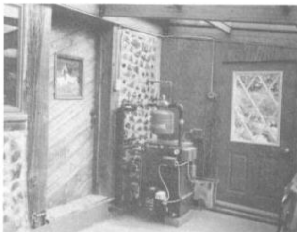
Illus. 16-5. The new oil furnace occupies a corner of the solar room.
