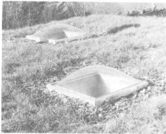
Illus. 15-1. Skylights, chimneys, and other roof projections should be surrounded by good drainage material, such as #2 crushed stone.
