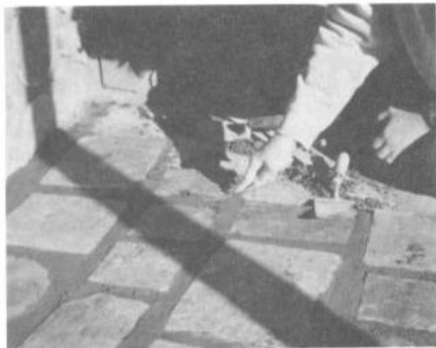
Illus. 14-6. Point the mortar between slates with a pointing tool made from a steel butter knife.
