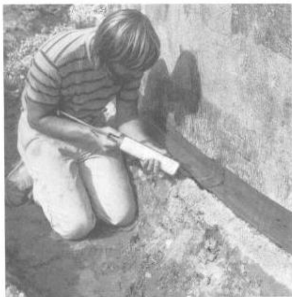
Illus. 9-1. The important detail where the footing meets the wall is sealed with a strip of Bituthene®.
