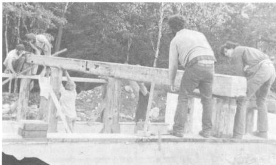
Illus. 7-4. The beam was then cantilevered over the north wall and positioned on the posts.
