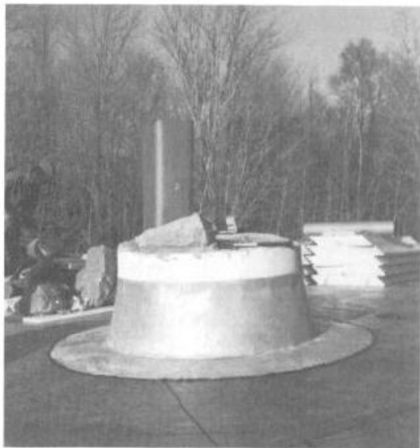
Illus. 9-7. A galvanized flashing cone was specially made for this cylindrical chimney.
