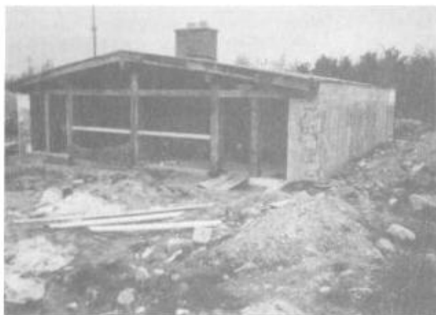
Illus. 16-4. Richard Guay's 40' x 40' Log End Cave during construction in 1980. The home is now fully earth-sheltered: berms on the north, east, and west sides; earth on the roof.
