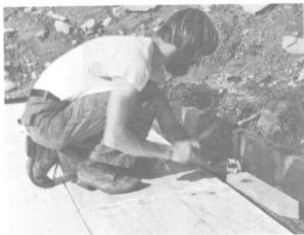
Illus. 8-8. Fascia boards were fastened by first nailing a 2 \times 6 plank along the edge of the roof, then nailing a scrap piece of economy-grade 2 \times 4 s on top of the plank. These two pieces provide a place for fastening the 2 \times 12 fascia.
