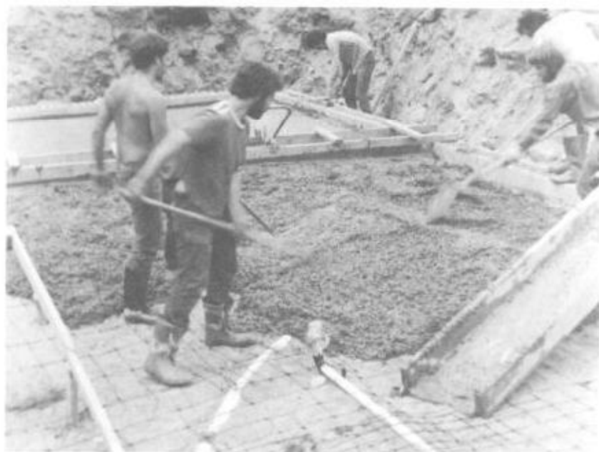
Illus. 5-11. It should be someone's job to make sure that the wire mesh is pulled up into the concrete.
