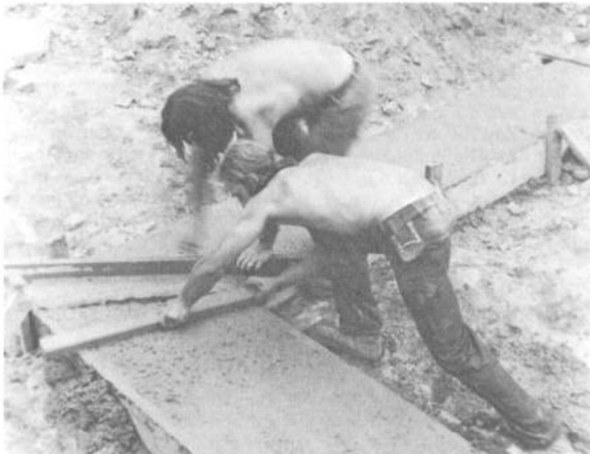
Illus. 4-12. The concrete can be screeded (made level with the top of the forming) with 2 × 4s.
