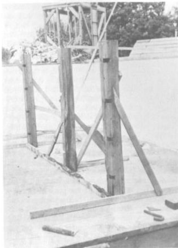
Illus. 7-3. After the internal posts are squared and cut, stand them up on their squares of roll roofing at the premeasured locations and shim, if necessary, to assure perfect plumb. The internal posts can be kept in place with a rough framework of 2 \times 4 s.
