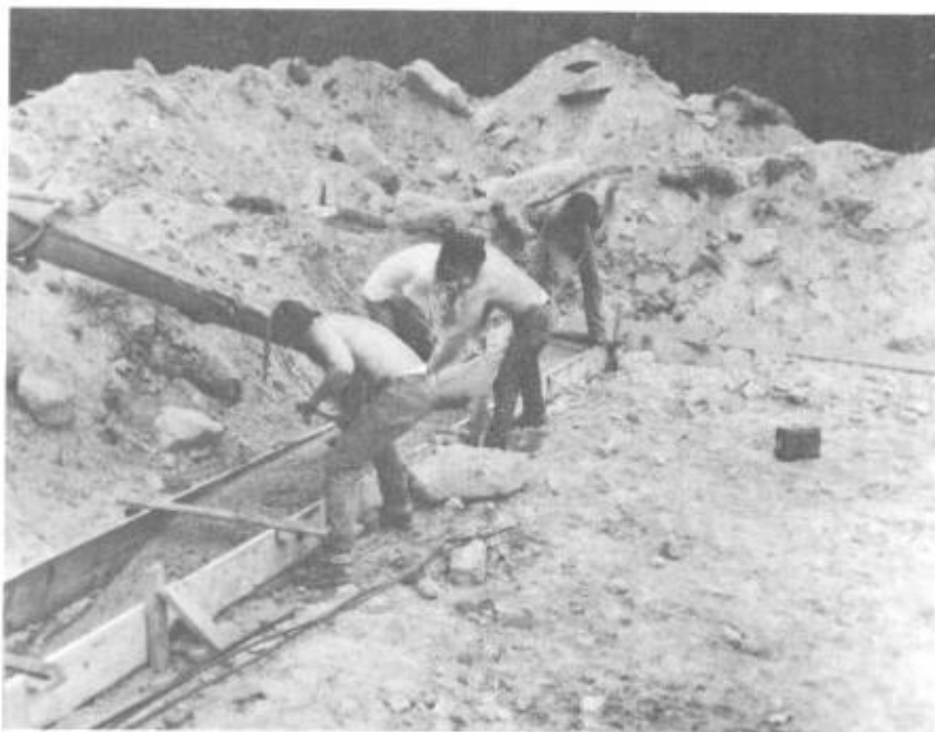
Illus. 4-11. A crew of four or five, each with a good strong rake, should be sufficient to draw the concrete around the footing ring.
