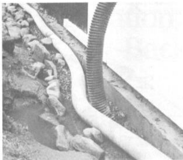
Illus. 10-2. The footing drain should be perforated-plastic flexible tubing, laid adjacent to the footing on a bed of washed 1" stone.
